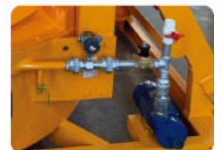
Pump & Flow Metering System
